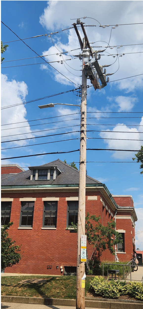
LED Cobrahead on a wooden utility pole
