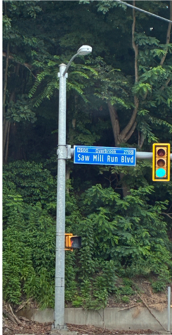
HPS Cobrahead on an aluminum lightpole
