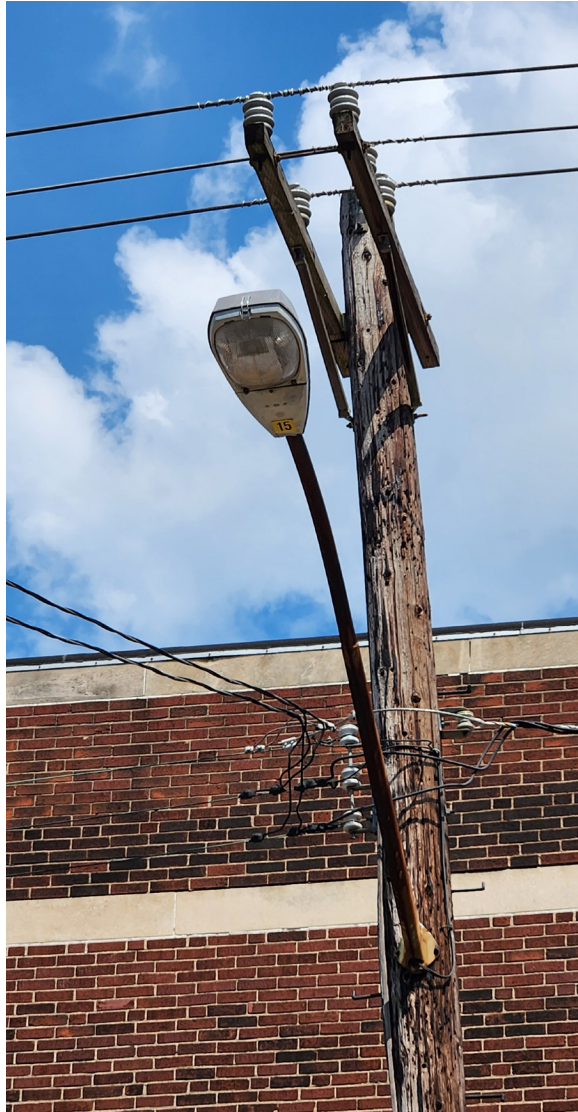
HPS Cobrahead on a wooden utility pole
