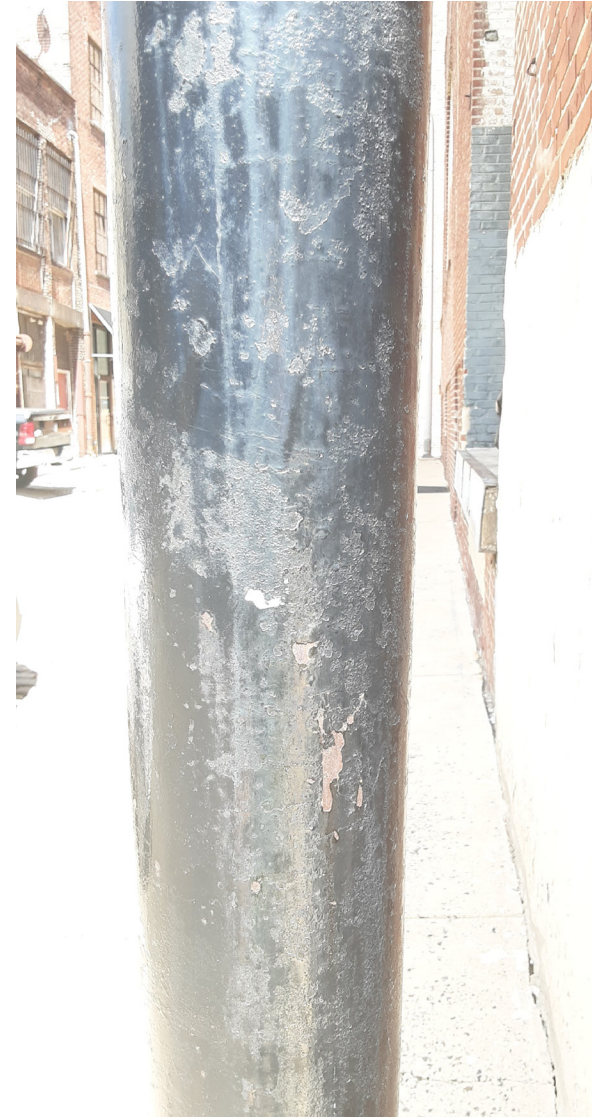
Typical trolley pole material and condition
